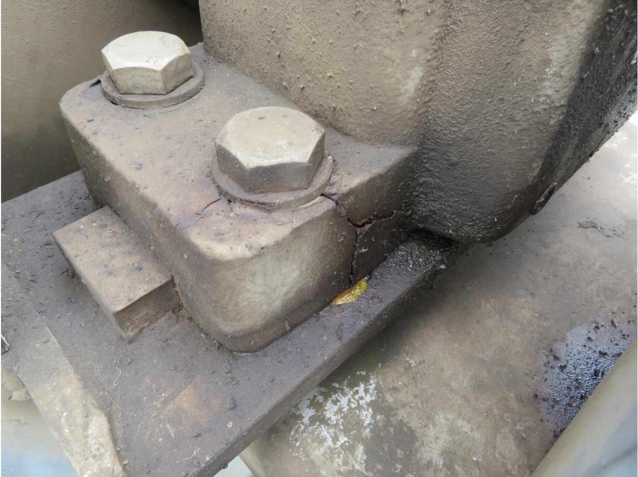
Photo 2. Close up of cracks.
